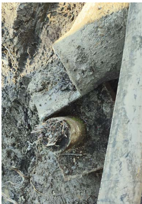
Some pipes were completely clogged with roots.
