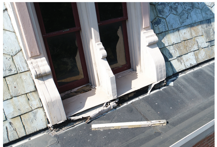
One of many sets of mansard windows that are badly in need of repairs.
